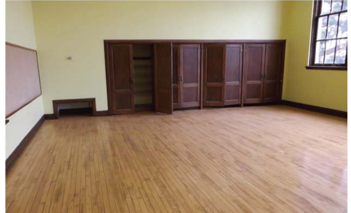
Carpeting has been removed and new windows have been installed in this former Central School classroom.
